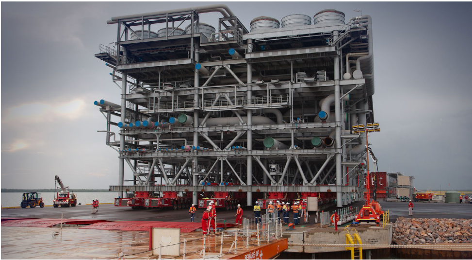
Figure 5 Module being unloaded at the MOF during construction of Ichthys LNG onshore facilities in 2016.
